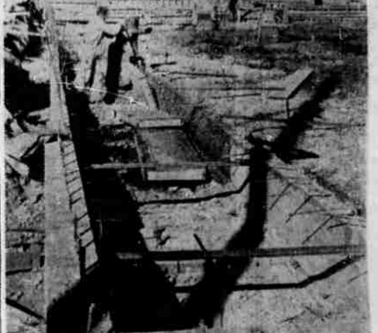
TAKING SHAPE — The Klamath County Courthouse addition is beginning to take shape after three weeks of construction work. Excavation has been completed, concrete footings have been poured and some plumbing is installed. James S. Hickey Inc. of Portland is the primary contractor on the half-million-dollar county project. A company spokesman said steel columns would be erected this week in preparation for the "lift slab" method of construction. The four-story addition is being built behind the present courthouse. It will be finished next summer.
