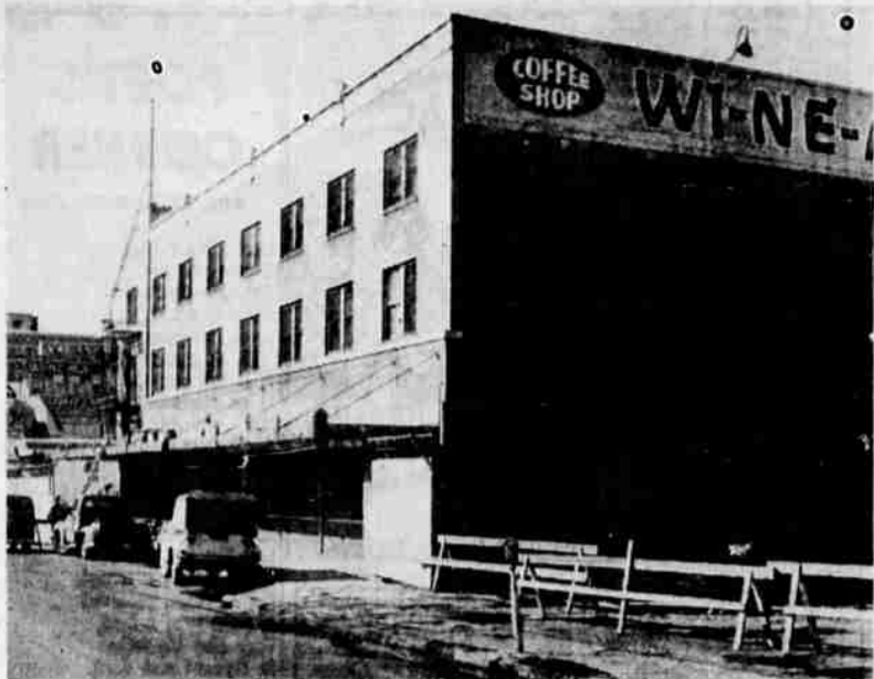
NEW FRONT — Bricklayers give a face-lifting to the front of the Winema as construction crews prepare for an office entrance addition on the north end of the Winema Hotel structure. Eventually, a three tiered motel arrangement will be constructed on this end of the hotel, but plans right now include building of an office and entrance structure. The hotel opened its 300 plus capacity banquet room several weeks ago, and remodeling work in the interior continues, including the relocation of the hotel lobby.
