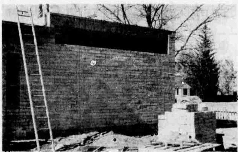
GOING UP — Duncan Construction Company, Klamath Falls, expects to complete the addition to the Merrill office of the Oregon Washington Telephone by late November. Manager Robert Graves says "This building is another way of showing our confidence in future growth of this area." Building will be completely modern.
