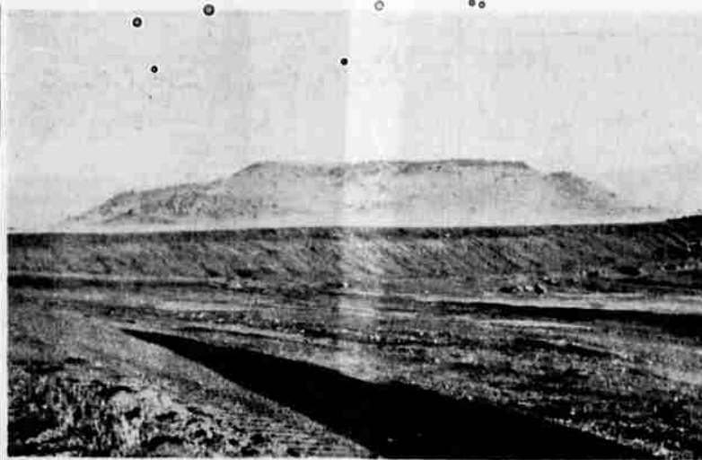
NORTH END — This is another portion of the land after digging and grading had been started for the reservoir.
