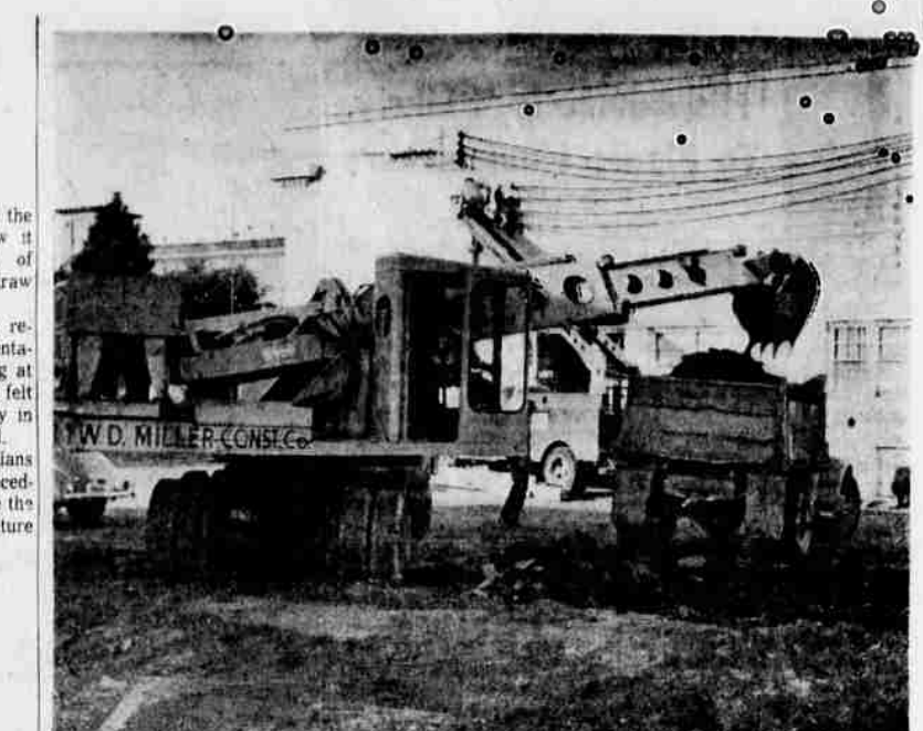
EXCAVATION BEGINS — Heavy equipment was digging and scraping behind the Klamath County Courthouse Monday as work began on the near half-million-dollar addition to the courthouse.
