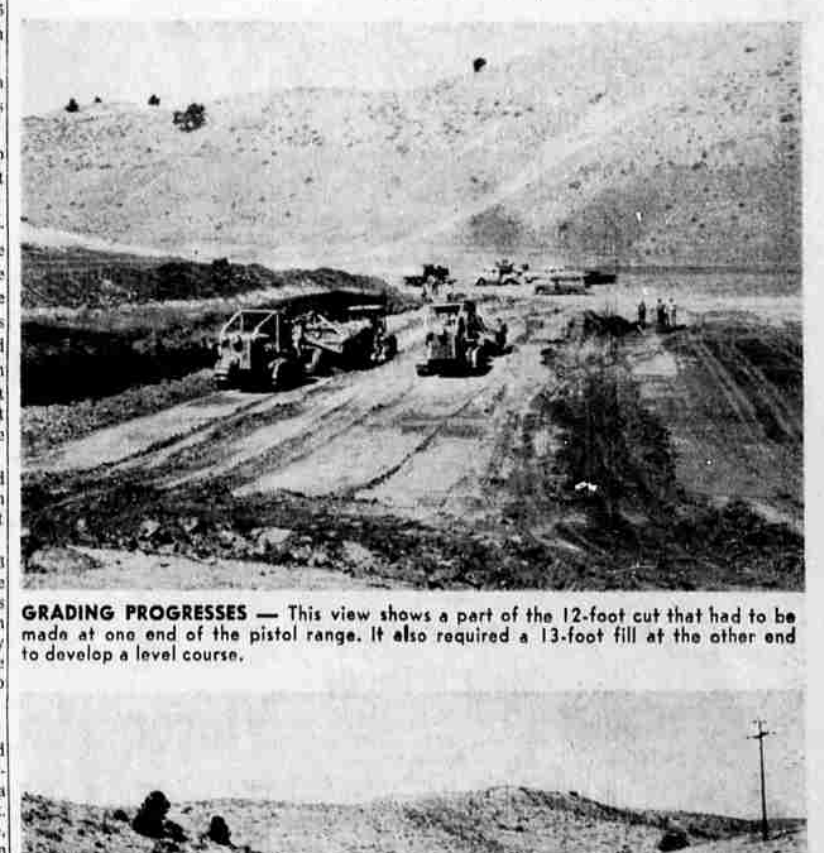
WORK BEGINS — This picture was taken during the first stages of the earth moving at the pistol course site. More than 12,000 yards of dirt were moved for the course.
