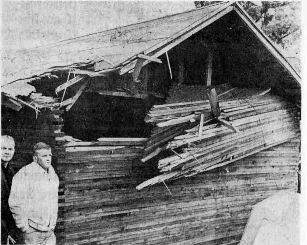
THIS IS THE CORNER of the garage adjacent to the H. H. McCann residence where the T-33 jet first struck. It clipped the garage a glancing blow and smashed on into the rear yard where it destroyed a play house and a storage shed.
