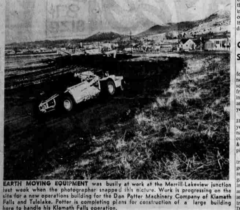
EARTH MOVING EQUIPMENT was busily at work at the Merrill-Lakeview junction last week when the photographer snapped this picture. Work is progressing on the site for a new operations building for the Don Potter Machinery Company of Klamath Falls and Tulelake. Potter is completing plans for construction of a large building here to handle his Klamath Falls operation.
