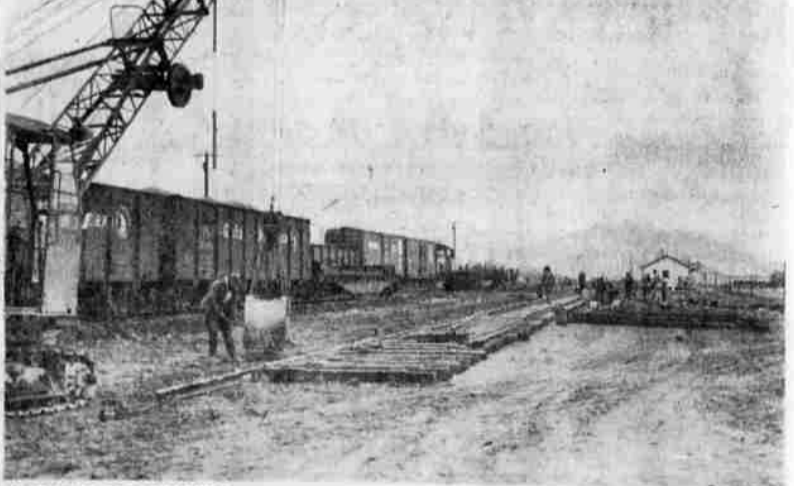
WORK IS PROGRESSING on construction of new facilities at the Great Northern Railway yards. The company is building four new classification tracks for blocking trains, and extending three tracks about 25 car lengths each, rearranging the switching lead. Crews have also leveled a slight hump in the switching yard. Ray Kizer Construction Company of Portland did the grading and earth-moving and GN crews are laying the new track.
