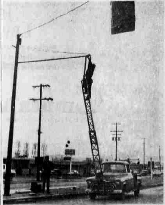
TRAFFIC SIGNALS at the intersection of South Sixth Street and Summers Lane were being mounted when the Herald and News photographer snapped this shot.
