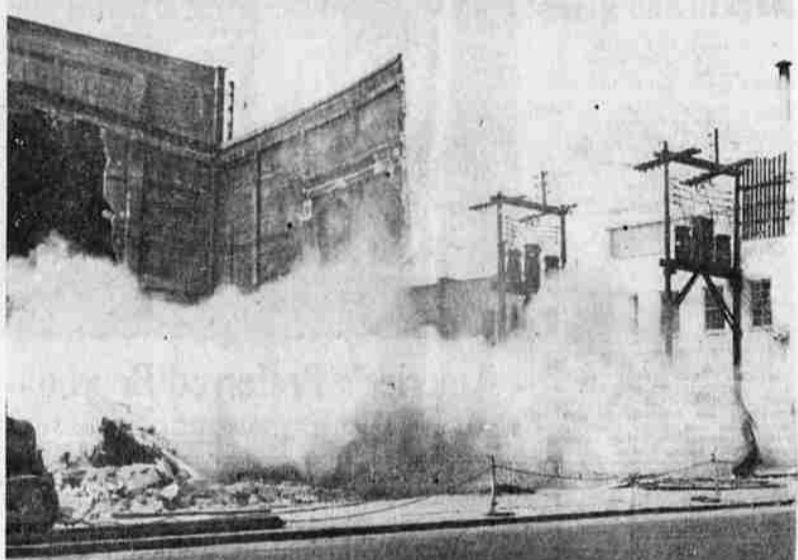
THE WALLS CAME TUMBLING down as demolition of the Pelican Theater moved rapidly ahead. In these views, the remaining portion of the sculptured front of the structure drops into dust. Top view, the wall begins to crumble, and at bottom, the dust billows up where the wall dropped amid the rubble. Plans still call for a parking lot to be ready for public use on this lot by April 1. The theater posed a problem to the Empire Wrackers of Santa Rosa, Calif., by its solid reinforced concrete structure, but it finally bowed to modern methods.
