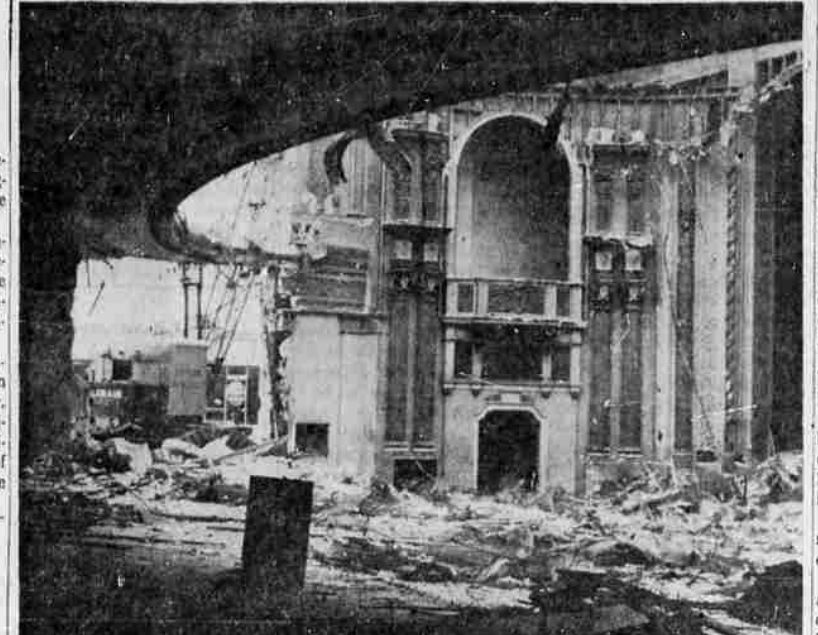
LOOKING LIKE the bombed out interior of a cathedral is this inside view of the Pelican theater as it continued to disintegrate into rubble in the smoothly planned demolition to clear the site for a parking lot. The reinforced concrete slows the rate of destruction, but everything is progressing as planned on this community landmark. Photographer Don Kettler got this unusual view late last week.
