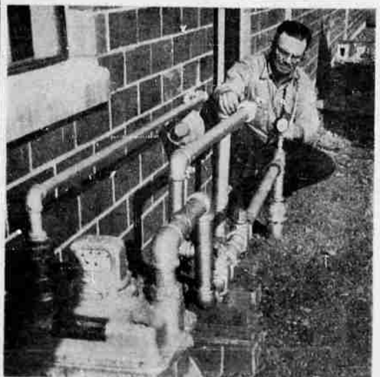
GAS INSTALLATION is shown at the city street department building, checked by Hugh Washburn, city employe. In foreground can be seen standby commercial gas installation which will be dispensed with by the sewer gas operation.
