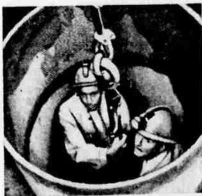
Only link to surface was pipe 42" wide, 40 stories deep. Heavy equipment was dismantled, lowered and reassembled on the cavern floor.
