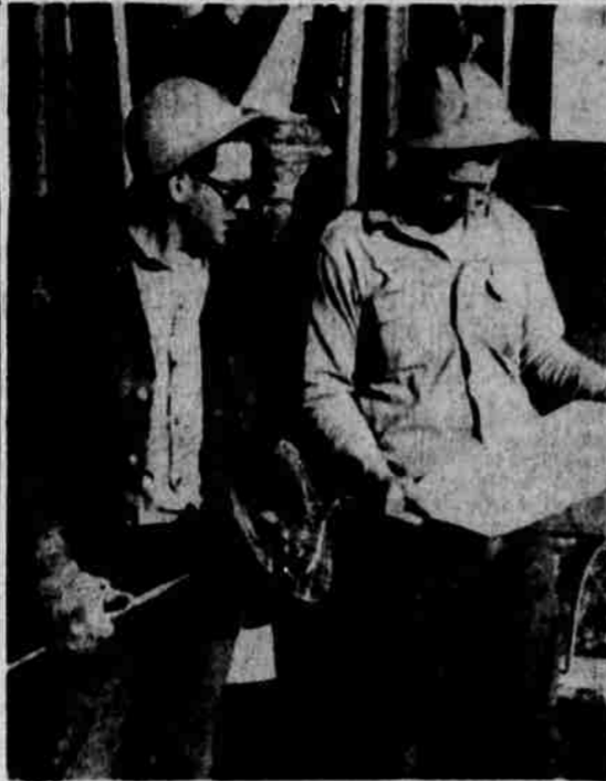
PHONE SERVICE in Fort Rock is coming close to reality as Pacific Telephone Northwest crews chisel through the frozen earth to place utility poles and guy wires. Ancel Rosecrans, left, and his brother, Gene, check specifications of their phase of the job. The former is holding a patented auger. Work was reported about one-third done last week. — Photo by Helen Parks
