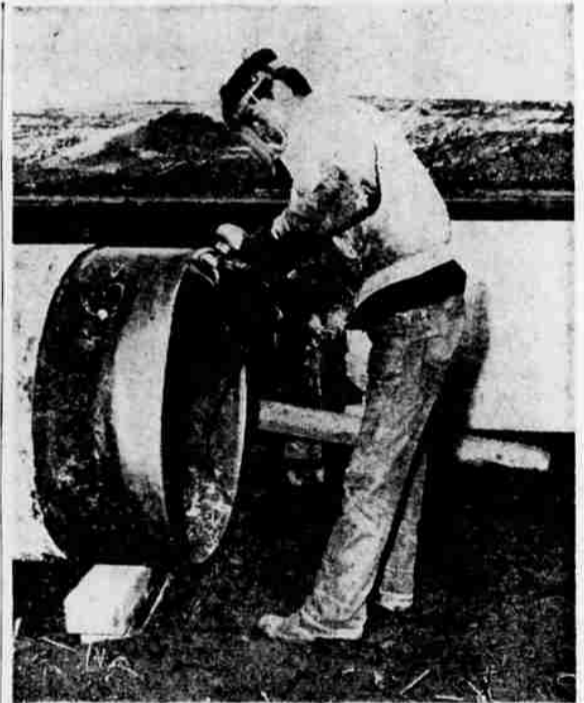
POLISHING AND SMOOTHING the pipe is the job of Don Brehm, shown here using an electric buffer on the end of a pipe section. This operation must be performed before two sections can be joined together.
