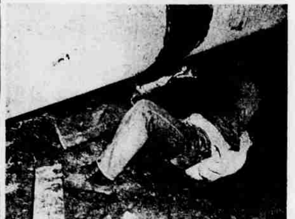
ALL SIDES OF THE PIPE must be buffed and polished so that joints can be wrapped and coated with a tar compound. Here, Franklin Barr taking his turn beneath the pipe with a buffer. This picture also shows why safety is stressed on the job. Most workers wear steel helmets on the job to protect themselves.
