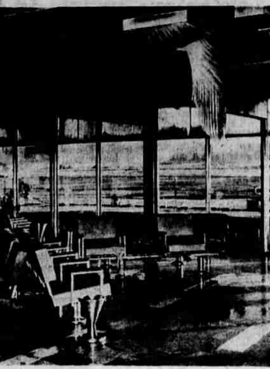
MOLTEN PLASTIC from light fixtures in the municipal air terminal swathed furniture and the floor with stringy gobs during a fire that scorched and smeared most of the new building Tuesday morning. This view is in the lobby looking out toward the parking area on the flight apron.
