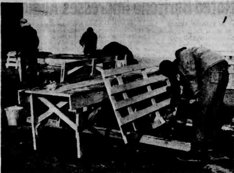
A DAP OF PAINT and a few well-placed nails will add up to new livestock pens at the Klamath County Fairgrounds. This renovating project is being performed by men in the Welfare Work Program.
