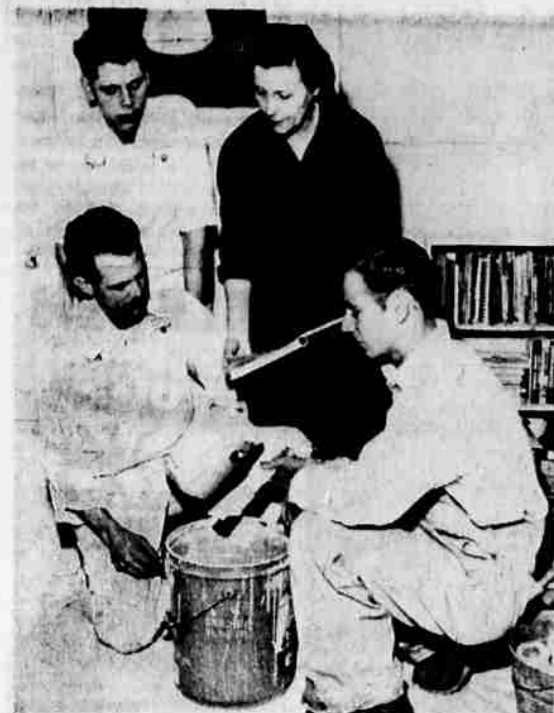
APPRENTICE PAINTERS Dennis Staley, top left, and Gerald Pacey, lower right, and their instructor, Henry L. Tayson, prepare to paint the Camp Fire Girls headquarters here. Meeting with them is Mrs. Naomi French, council executive.
