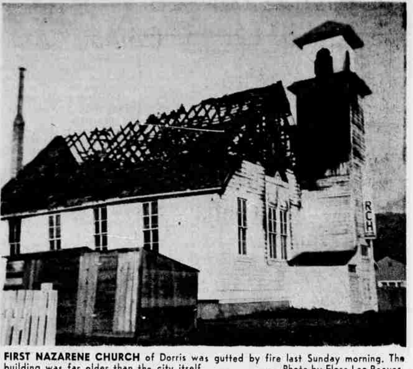
FIRST NAZARENE CHURCH of Dorris was gutted by fire last Sunday morning. The building was far older than the city itself.
