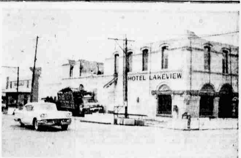
A LAKE COUNTY LANDMARK since 1901, the Hotel Lakeview is being partially torn down for remodeling into a restaurant, supper club and lounge. Ritter and Sons, a Salem firm, has almost finished demolishing the two upper stories and plans call for reopening under a new name about May 15. The new operation will continue under the management of Robert Ogle, son of Mr. and Mrs. Lloyd Ogle, who have owned the hotel since 1928.
