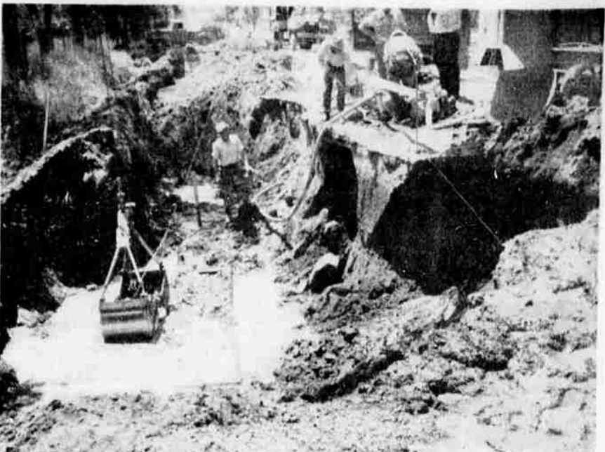
THIS CANYON on Homedale Road began as a routine pipe zone. Sides sluffed in, leaving a hole eight feet deep, 35 feet wide, and 300 feet long. One weekend a broken water main flooded the hole, creating "Lake Homedale." It took a day to pump it dry. (See story Page 3-A).
