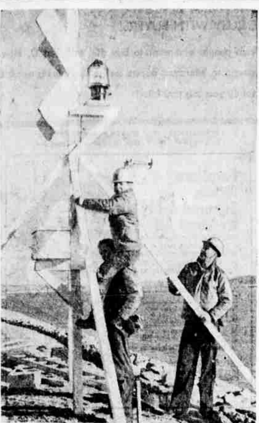
UP HE GOES!—Coast Guardsman Jerry Meyer is at it hammer and tongs as he climbs onto the shoulders of Albert Reimert at Memphis, Tenn. He's about to nail the braces of the Robinson Crusoe Light being installed along the Mississippi River. It was set up to guide towboats working on the curve-straightening of the river channel.
