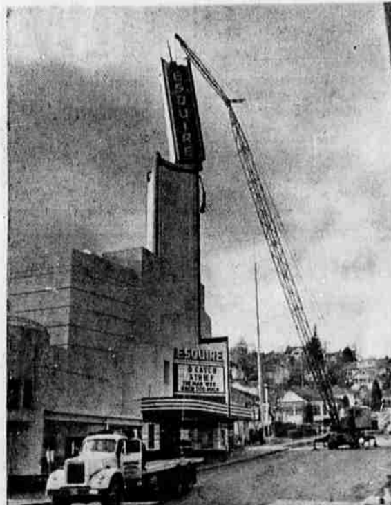
A CITY LANDMARK came down on January 8 after wind had damaged its supports. The sign atop the Esquire Theater is shown being lowered to the ground to prevent an accident. After repairs, the sign was hoisted back into place on June 24. A strong wind caused the sign to sway dangerously during a two-day storm that swept the area.
