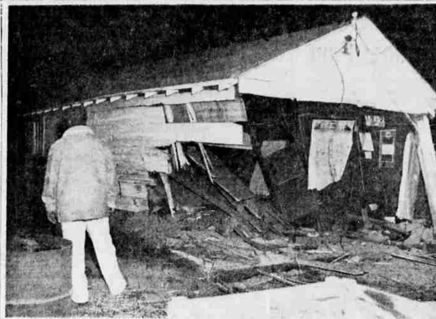
SURVEYING THE DAMAGE that his automobile caused to the office building at the Richardson Lumber Yard on Spring Lake road is AIC Orlando Thomas, Falcon Heights. He was southbound on Spring Lake Road, and state police report that his automobile apparently went out of control at the curve. The car careened over a ditch, struck the building causing considerable damage, and coming to a halt in the middle of the lumber stacks. Thomas suffered a slight cut on the forehead. The investigation of the accident is continuing.
