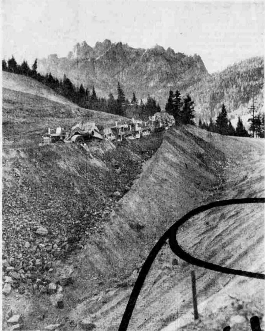
JAGGED CASTLE CRAGS tower above this four mile stretch of freeway south of Dunsmuir. A fleet of cat-drawn scrapers, each hauling 20 yards of earth, is literally lifting a new road 40 feet above the present highway where it threads its way through the Sacramento River Canyon between Redding and Dunsmuir. Gibbons and Reed are contractor for this portion of the road, first mile of which will be open to traffic about November 18.
