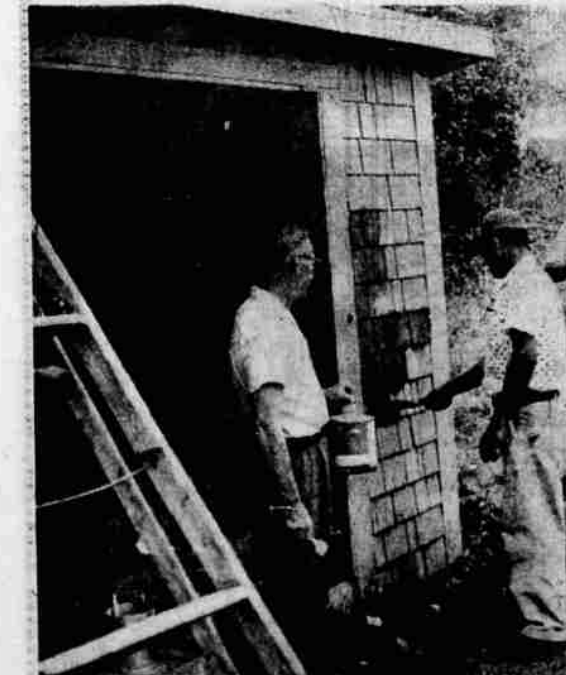
SCHOOL BUS SHELTERS are being readied for the term opening by Weed Lions Club members. Original building of three shelters was a Lions Club project several years ago. A fourth was built by a neighborhood group and placed at Fourth and Walnut and is being maintained by the club. Over 300 Weed students ride the bus and make use of the shelters. — Photo by Gaynor
