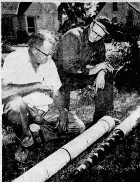
THE KEY to Fred Lewis' sewer pipe laying machine is the auger that fits inside a pipe. Joint lengths of pipe and auger are bored into the earth together. Looking it over are Maurice Gunderson, left, sanitary district engineer, and Lewis.
