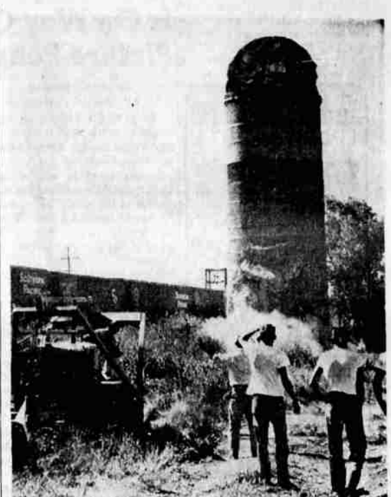
AN OLD LANDMARK came tumbling down Tuesday afternoon when equipment of Graham Brothers was used to pull down this sawdust burner on East Main property owned by Long-Bell Division of the International Paper Company. Exact date of construction of the burner is not known, but Long-Bell officials estimate it was built in about 1905. The burner was torn down to clear the lot which has been sold to a Klamath Falls automobile dealer.
