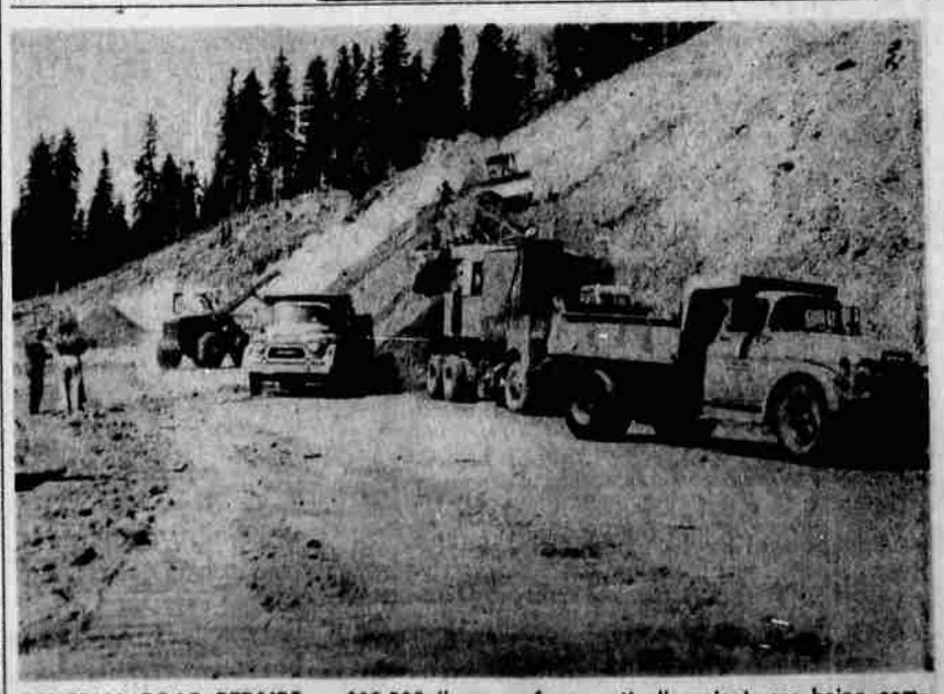
REMEDIAL ROAD REPAIRS, a $32,500 "ounce of prevention" project, are being completed on a mile-long strip of Everett Memorial Highway near Mt. Shasta. Slopes are being pared down to prevent dislodged rocks from rolling onto the highway. Freezing and thawing and heavy rainfall in this area make falling rocks an extreme traffic hazard. The Bureau of Public Roads is providing $25,000 for the work and Siskiyou County the balance. — Photo by McKinney
