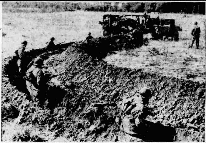
NO MORE SHOVELS? —Army mechanical ditch digger is tested at Ft. Belvoir, Va. It could scoop out battlefield trenches and fox holes in minutes. It can dig a trench four feet deep and two feet wide at the rate of 12 feet per minute.
