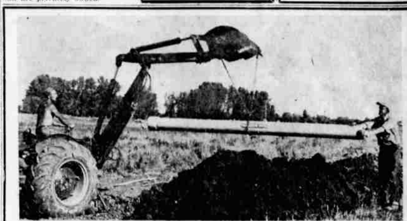
C. A. BUSH, Klamath Falls Digging Contractor, is shown installing a section of 8" Johns Manville Transite Sewer Pipe for a local sub-division project. Supplier for the pipe is the South 6th Street Steel Co.
