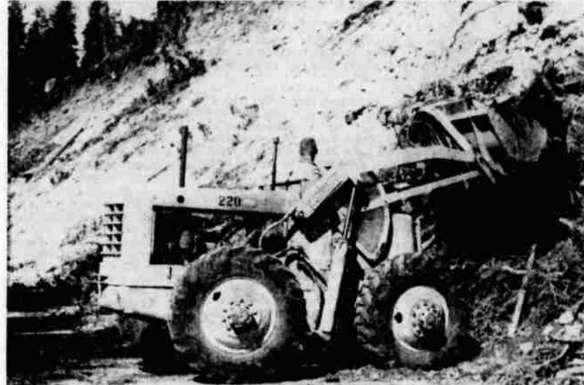
ROCK SLIDES that caused concern to motorists on the Everitt Memorial Highway and complicated snow removal to keep open the road to the Mt. Shasta Ski Bowl are being eliminated by terraces set along the slopes with fences to stop rocks at these points. Crews and heavy equipment of both the Bureau of Public Works and Siskiyou County are tearing down the slopes which cascaded rocks onto the road. —Photo by J. O. McKinney
