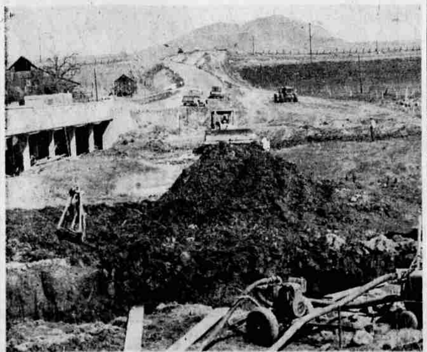
WORK ON THE NEW BRIDGE across the Shasta River a mile and a half west of Montague is moving rapidly ahead. Here, bulldozers of the Bos Construction Company of Berkeley, are trenching and preparing the ground for the cement structure. It will be a 120 foot span with two 14-foot lanes, and will cost approximately $107,518. The old bridge at far left will be torn down. — Photo by Don Kettler
