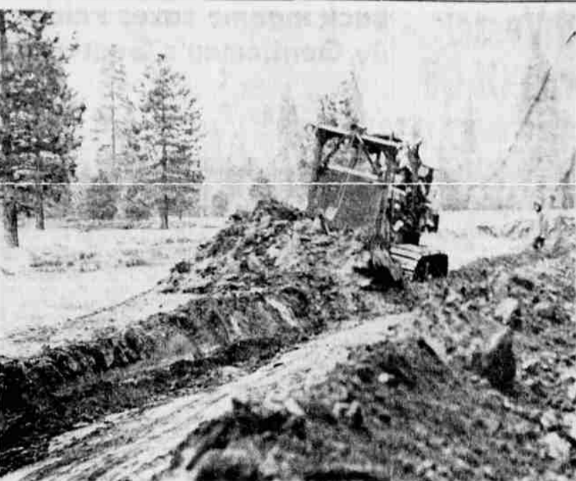
A STREAM POLLUTION problem created by Ash Creek flowing into the McCloud River is being cleared up. Here, Bud Parker operates a bulldozer. Parker donated his time for the job. New channels were made in the sandy flat and a dyke built to store the muddy flow from the slopes of Mt. Shasta. Evaporation and seepage should restore the crystal clear water in the McCloud River. This is a project promoted by the McCloud Fish and Game Club.
