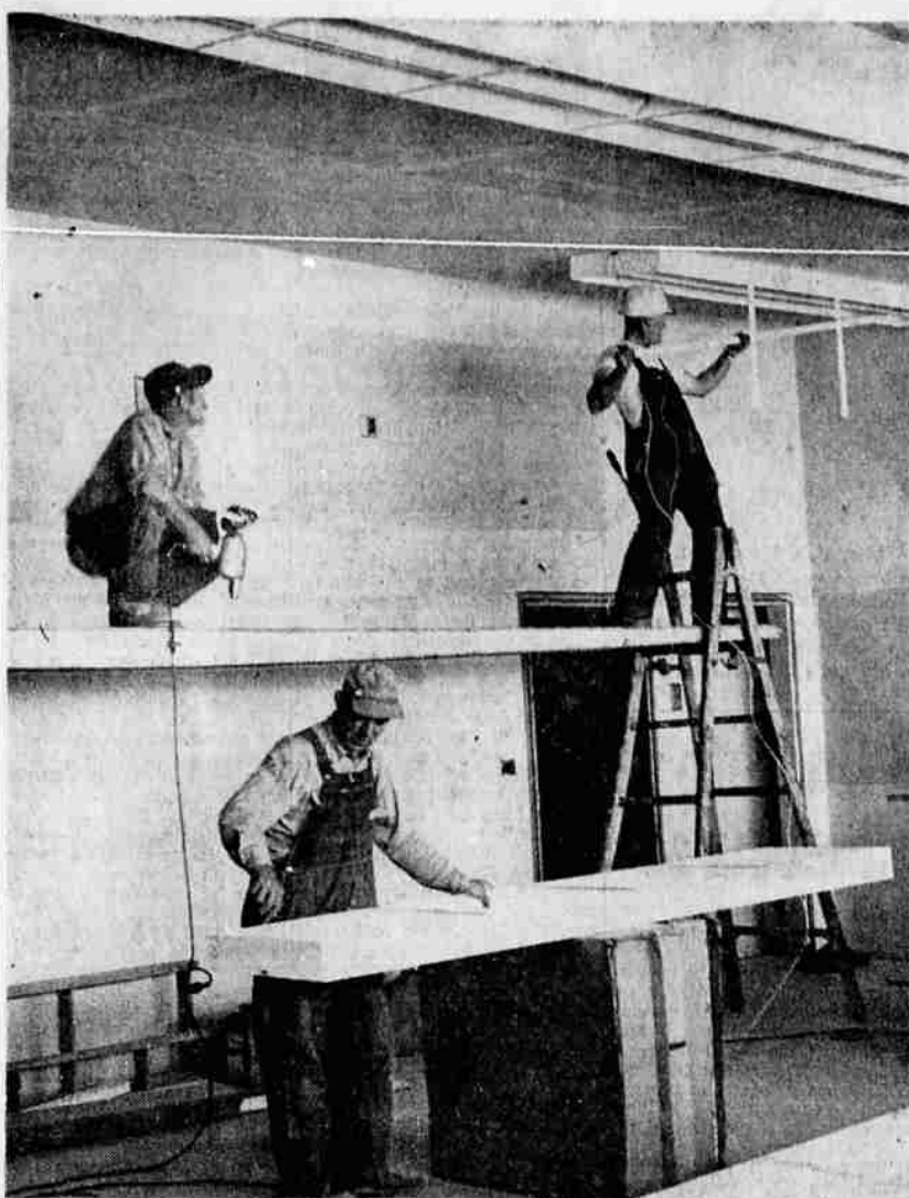
PROGRESS on the new Weed High School has moved ahead with no interruptions. Here is a shot of the interior of one of the seven general classrooms. Workman on the ladder at left is Thomas Lotz. Lee Musckett puts in a light fixture at right, as George Brewster works on another frame below. A. J. McMurray Construction Company of Yreka is contractor for the $595,000 school plant. Work is on schedule for the 1960 fall term opening. Architect is Howard Perrin, Klamath Falls. —Photo by Don Kettler
