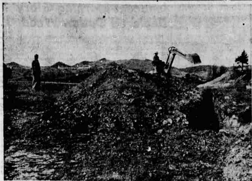
CONSTRUCTION was started Thursday on a new shopping center to be located on a seven and one half acre area on Shasta Way and Alameda near the "A" Canal. John Fehlen, resident of Klamath Falls for 26 years, said all building construction will be of pink pumice tile. First businesses expected to occupy the shopping center will be groceries and meats, drug store, barber shop, electrical appliance store and a restaurant. Some lots will be sold for individual businesses. Fehlen, left, looks on as shovel operator Lewis Walker digs sewer ditch.
