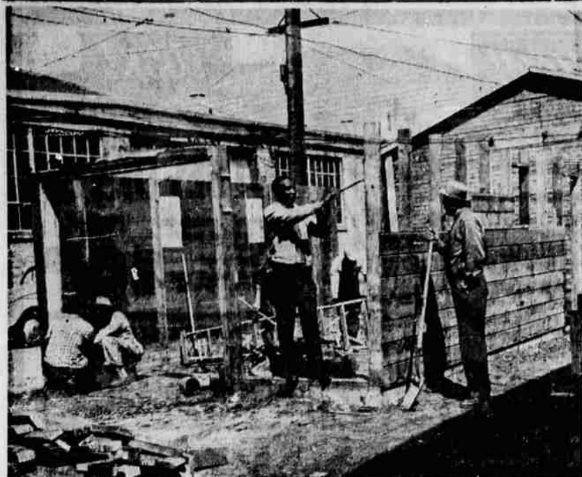
A GARAGE at the rear of the Klamath Falls Gospel Mission, 823 Walnut Avenue, is being torn down to make way for a new addition to the building which in one year has been outgrown. The addition will include a basement and two stories to include a dormitory to accommodate 50 men on the top floor, a reading room, showers and lavatories. The present kitchen at the front of the basement will be moved to the rear of the new section. The 40 by 28 structure will be built of pumice tile blocks. The addition is being started with a small cash fund. All work possible will be done by men who stop at the mission. Anyone who cares to share in helping finance the building in any way may contact a member of the board of directors, John Pederson, right, mission superintendent or Jack Wright, with crowbar, assistant. Men in rear are not identified.
