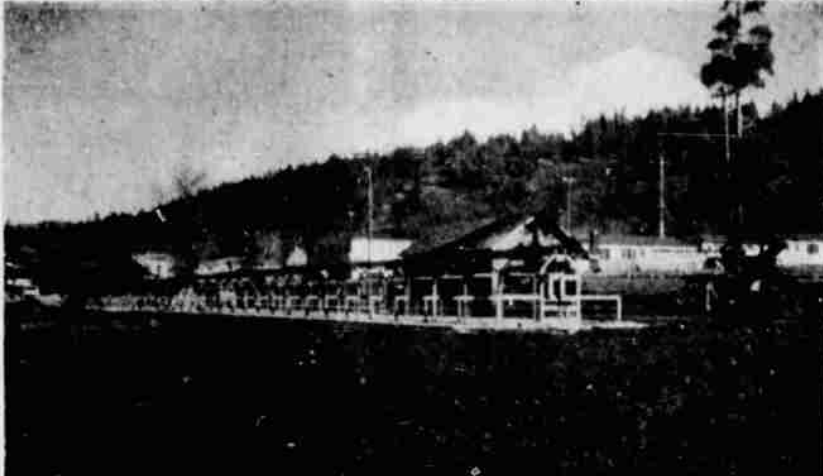
A MOSELEY SORTWELL LUMBER SORTER is being installed at the Ralph L. Smith Lumber Company Mill in Mount Shasta by the Irvington Machine Works of Portland. The automatic machine will sort, according to length and width, 360 board feet per minute and stack in 26 different combinations. Seven men are replaced by the automaton and they will be used to expedite the flow of lumber to the big 326-foot installation. Robert Kohn, superintendent of the Smith Company, states that more lumber at the same cost can be handled by the mill.
