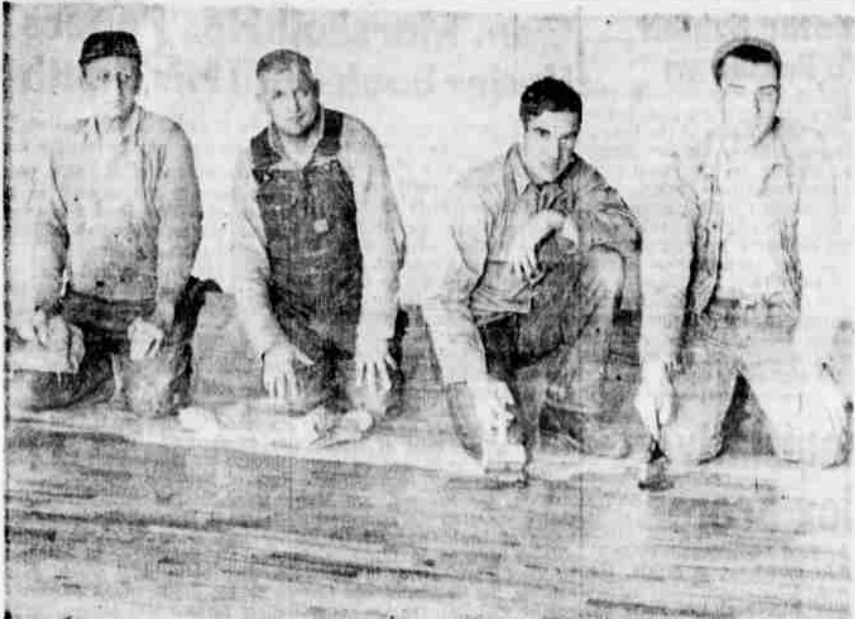
FINISHING THE NEW FLOOR at the Fort Rock Grange Hall at their recent work day are grange members, from the left, Merlin Black, Edwin A. Eskelin, Master Harold Miles and Earl Lyman. Most materials were donated by grange members. The job has required many hours of volunteer labor and at least a dozen helpers in addition to these men, took part in the improvement. —Photo by Bill Parks
