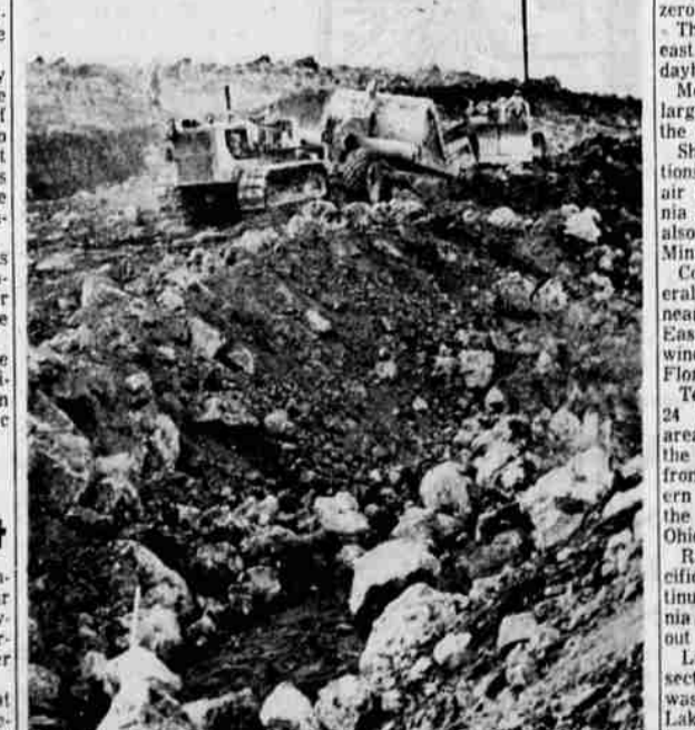
THE APPROACHES to the California overpass are being routed out by earth-moving machines which are encountering hard going in the rocks, as witnessed by this picture. Much of the actual grading has already been accomplished. Completion, including structures and paving, is expected in late 1959.
