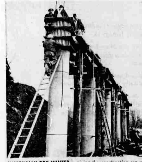
UNUSUALLY DRY WINTER is giving the construction crews along the west side bypass a helping hand. Here, they are moving rapidly ahead in building the supports for the bridge that will span the Nevada Street area and provide an interchange at this spot. The Tom Lillebo Construction Company of Reedsport has the contract for the bridge across the A Canal and the overpass across California Avenue also.
