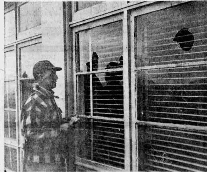
HERE ARE SOME of 30 windows in KUHS broken by vandals in a wave of anti-Christmas enthusiasm this week. Inspecting the damage is Walter Hamblin, a maintenance man at the school. Hoodlums went out of their way to leave their destructive mark at KUHS and at Conger School, heaving rocks, bricks and concrete blocks as heavy as 25 pounds. They added to their moronic glee by heaving rocks through more than half a dozen car windows, city police reported.
