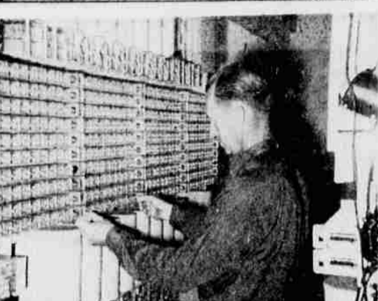
EDWIN T. ASCHOW, supervisor for Western Electric Company from Sacramento, pulls the last blocking tools out of line relays. This marked the completion of installation and the starting operation of the new dial central telephone office in Montague, which went into operation on October 17 at noon. Aschow supervised the installation of the entire new system in the Montague office. — Photo by Dow
