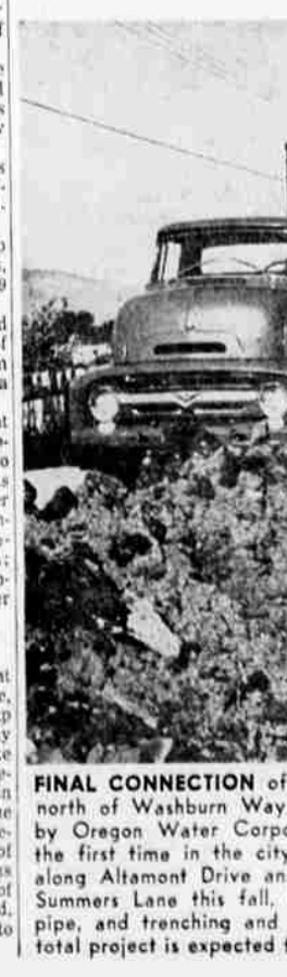
FINAL CONNECTION of a 1,300-foot pipeline connecting a million-gallon reservoir north of Washburn Way with south suburban water mains was completed Wednesday by Oregon Water Corporation crews.
