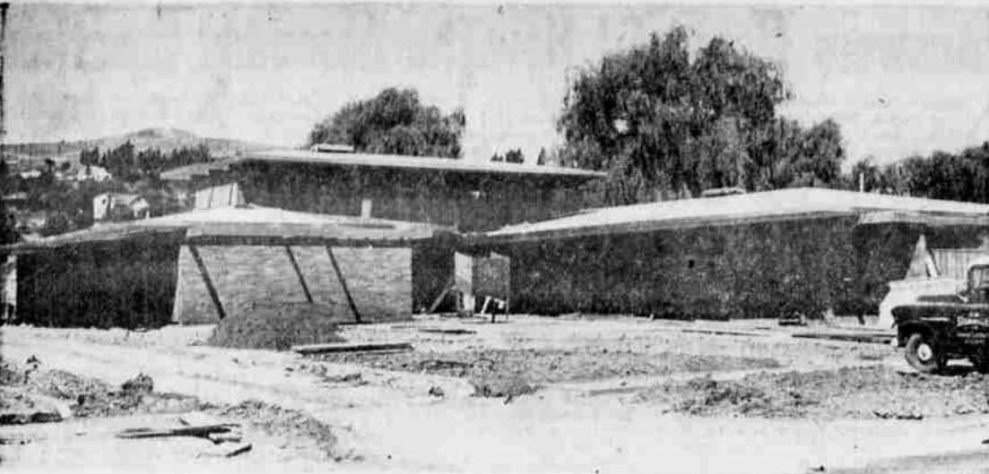
CONSTRUCTION of the new Klamath Medical Clinic at 1905 Main Street is going ahead on schedule, according to Glenn Evans, business manager for the clinic partnership. General contractor is John M. Steinmueller Jr., of Eugene, and completion is slated for the end of this month. Moving into the new location is set to begin on September 2 and should be finished by September 5, Evans said. The new building will provide offices, laboratories and clinics for five physicians and two dentists.
