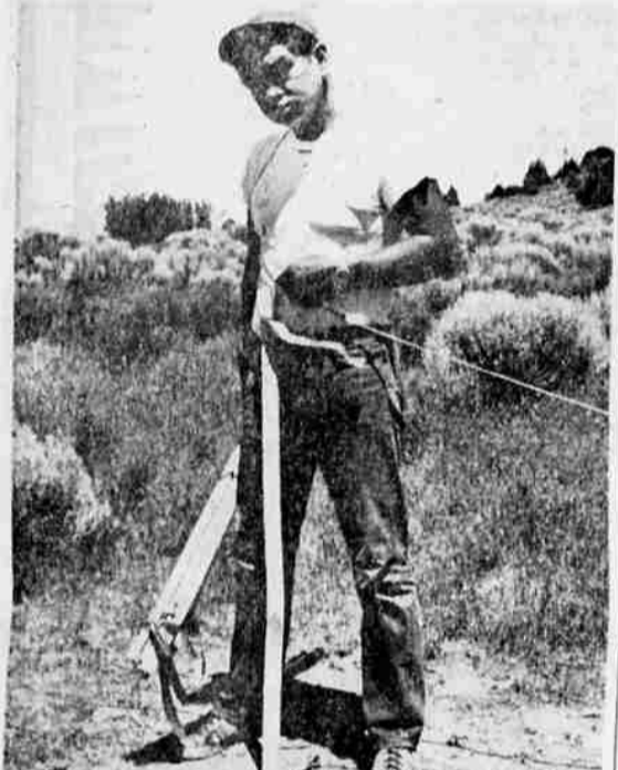
BILLY SUNDAY is acting as chairman on the Klamath Agency road construction crew which is building a new 12-mile two-lane gravel road to replace a one-lane dirt road on the reservation that is virtually impassable in winter. The new road will be an all-weather road and starts at the town of Sprague River, ending about four miles north of Beatty. The "chain" in use is actually a 100 foot steel tape. Formerly surveyors used a chain to measure distance, and after the advent of the steel tape, the name chain still persisted. —Nelson Sharp Photo
