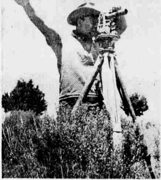
CLIFFORD CASE of Klamath Agency, a member of the Siletz Indian tribe, is shown waving the chainmen on line on a road-building project on the Klamath Reservation. Twelve miles of new road starting at the town of Sprague River and continuing east along the base of the tableland, on the north side of the river, and terminating at a point about four miles north of Beatty are now under construction. When this picture was taken, the survey was being made to set stakes for fences on either side of the road right-of-way to keep stock off the road. —Nelson Sharp Photo
