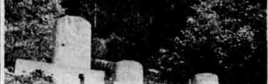
NEW WATER SUPPLY for the city of Mount Shasta will feature the use of concrete and metal conduits to assure adequate anti-contamination control of the water supply. Shown here is a concrete structure at one of the 15 big springs that will supply Mount Shasta.—Photo by McKinney
