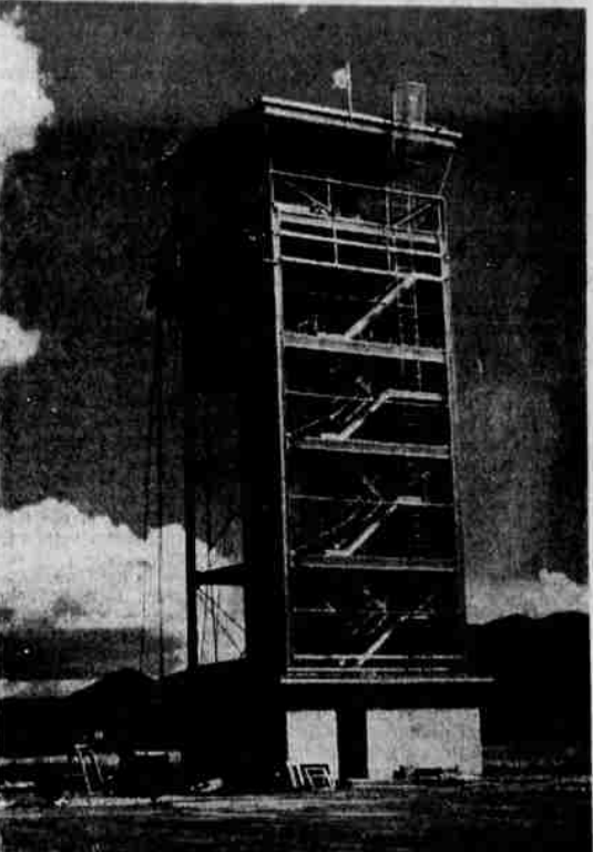
THE CONTROL TOWER at Kingsley Field is now about 50 per cent complete, and should be finished by mid-July, the Navy, which is supervising the construction, reports. Begun in February, the tower is being built by Thompson and Geogerson, Inc., Portland, for an estimated $90,900. Sixty-eight feet high, the tower will be shared by traffic control personnel of the Air Force and the Civil Aeronautics Administration, to control both civil and military traffic in this area.
