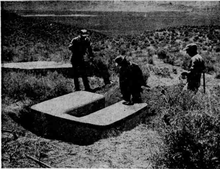
OREGON Game Commission personnel are pictured installing one of the new type plastic guzzlers for quail and dove in some of the arid regions of Oregon. The pictured water guzzler for the brush bound birds is in the Lakeview area. —Game Commission Photo
