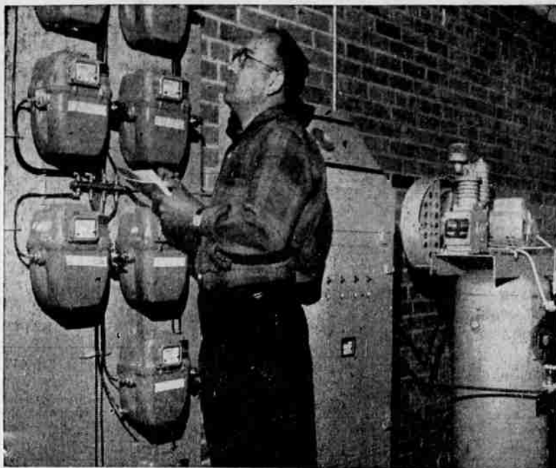
A BETTER JOB of maintenance will be possible with this new pumping system which will pump dried air into the telephone cables to spot possible leaks. For Pacific Telephone it represents "a stitch in time saves nine." Daily checks are made on pressure in the cables, and a loss of pressure sends repairmen on a search for a leak that could cause loss of service.
